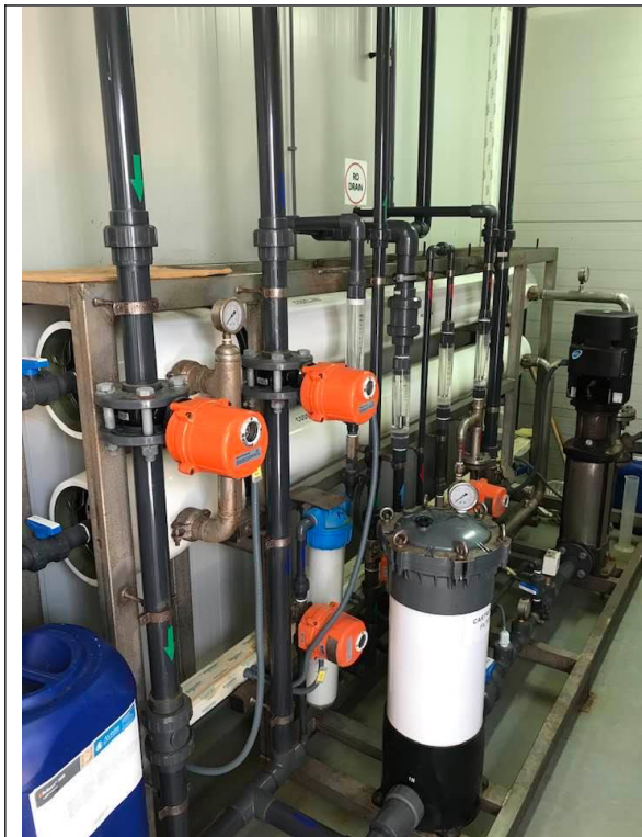
Reverse osmosis desalination unit at EJUST campus, providing safe and free drinking water
